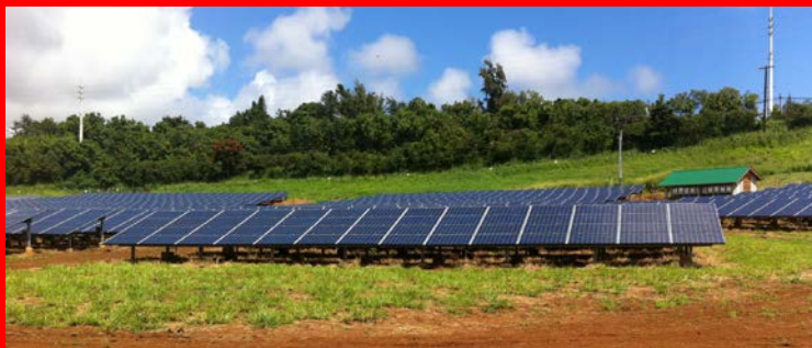
1.2-MW PV array on Kaua'i. Photo by Jamie L. Keller, NREL 21774
