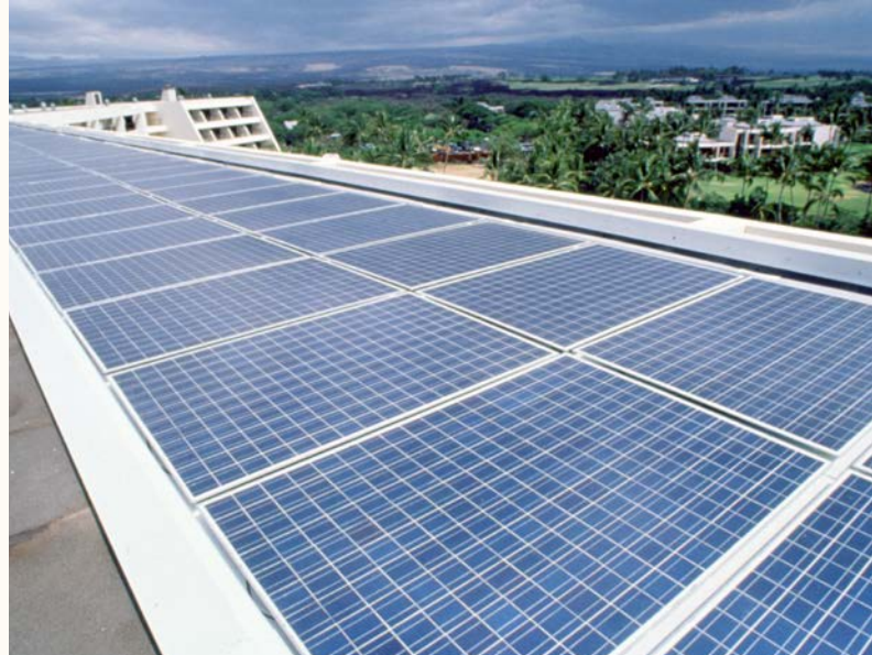
The rooftop solar PV on Hawai‘i’s Mauna Lani Bay Hotel generates 75 kW of electricity. Photo from SunPower, NREL 06430
