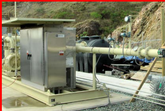
A landfill-gas-to-energy conversion system at Bovoni Landfill on St. Thomas will bring the USVI one step closer to meeting its clean energy goal. Photo from Dan Buchanan, VIEQ, NREL 2017.
